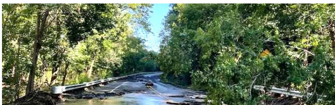
Route 29 was just one of the roads in Kingwood that were severely damaged by Ida's floodwaters. Photo Credit: Rose Frey
